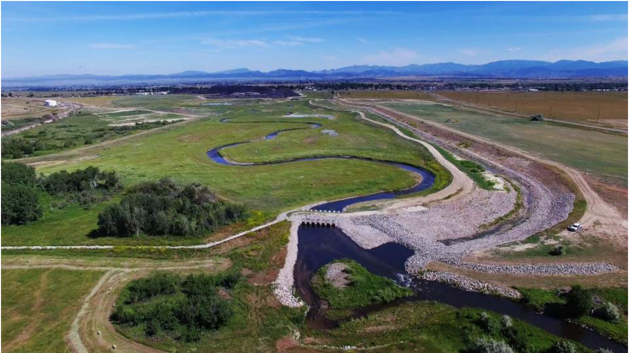
The Prickly Pear Creek realignment – completed by the Montana Environmental Trust Group and its contractor Pioneer Technical Services, and recognized with a 2019 national award in engineering excellence – moved 1.25 miles of Prickly Pear Creek in East Helena, Montana away from a massive, contaminated slag pile and created wetlands, wildlife habitat, and conservation land.
